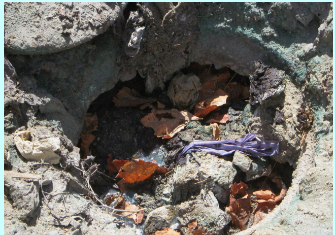
Exposed and full cesspool tank opening
