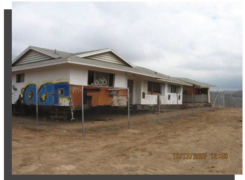
Summary abatement was necessary on this substandard structure
